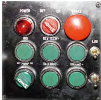
Electric control panel
